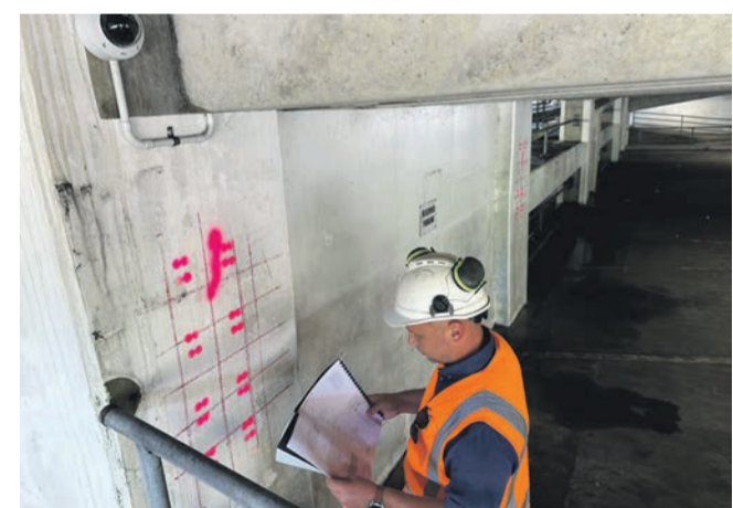
NPDC Senior Infrastructure Project Manager Joel Richardson checks the proposed drilling points on a column in the Downtown Car Park.
